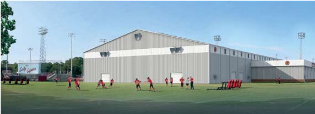
Construction of this indoor practice facility was slowed earlier this spring by frequent rains. When it's complete, it will be used by all UL Lafayette athletic teams.
