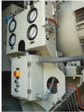
This Saturn diesel turbine generator can power about 700 homes.
