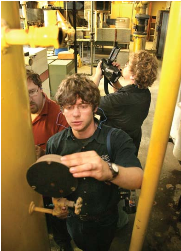
In the TABASCO® factory, from left, Blakeley Blanchard and Aaron Artigue check the air compression system, while Ryan Kelley takes readings with a thermal-imaging camera.
